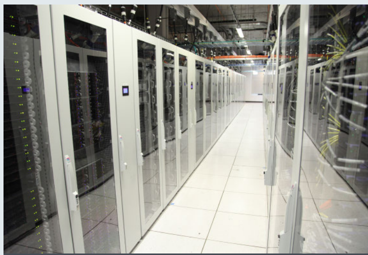
The NCI Genomic Data Commons is housed at the University of Chicago Kenwood Data Center.
