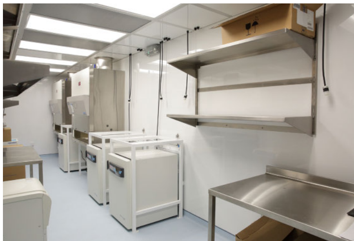
Interior of CC Trailer 10B
