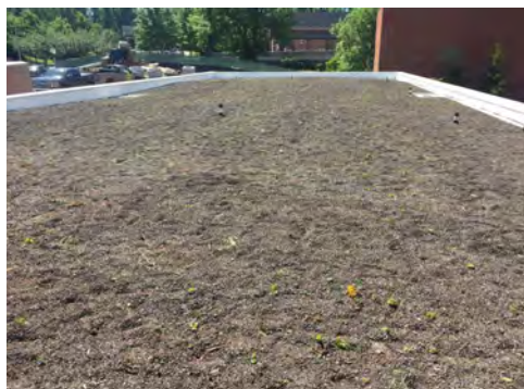
In May 2017, the green roof atop the Northwest Child Care Center was barely worth the title, just getting underway.
