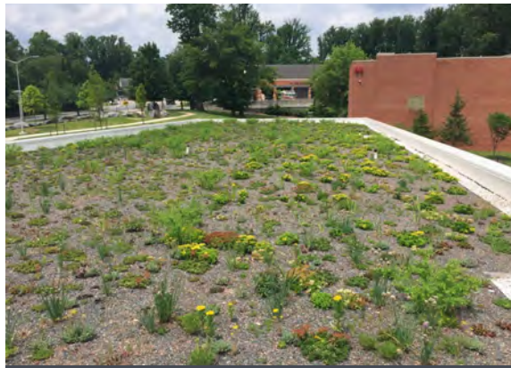
Installed in spring 2017, the green roof on the Northwest Child Care Center shows growth in June of this year.
