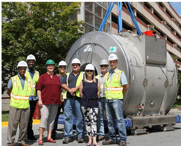
The team involved in the 7T magnet renovation and installation project included (from l) Mesfin Medhin, construction management personnel mechanical inspector; Aaron Burroughs, facility operations and maintenance staff; Dr. Joelle Sarlls, NMRF staff scientist; Seung Yang, project manager, Healthcare Design Builders; Chip Gavin, senior project manager, Siemens Healthineers; Joellyn Stolinski, NMRF MRI technologist; Dave Sweeney, director of operations, Healthcare Design Builders; and Daniel Lid, ORF project officer.
