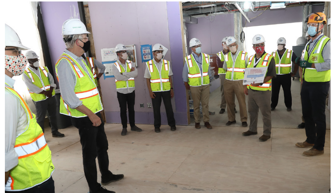
Inside the CARD, NIH director Dr. Francis Collins (third from l) gets a briefing on construction progress.
