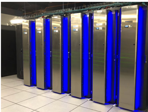
Supercomputer Biowulf uses a massive cooling system to maintain the appropriate temperature for its 99,000 cores.
