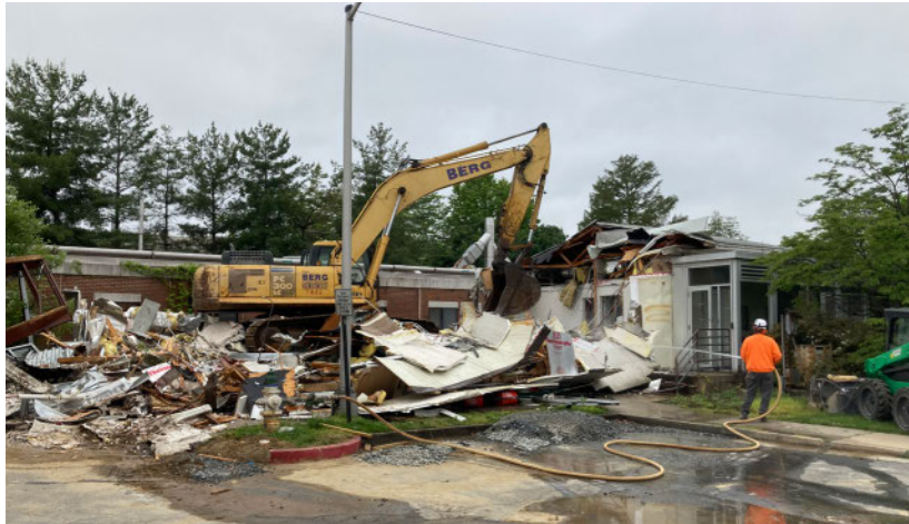
Days later, it took barely an hour for Bldg. 18T to turn into a pile of rubble.
