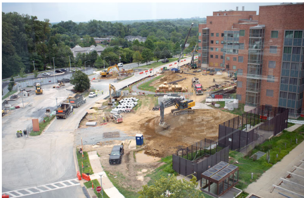
Viewed from the MLP-14 garage on Aug. 3, construction of the Clinical Center's surgery, radiology and laboratory medicine wing is well underway.
