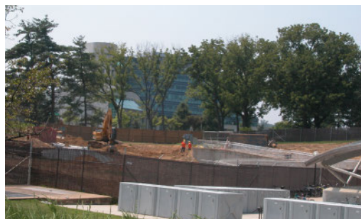
A new NIH Gateway Center is under construction near the Medical Center Metro Station.
