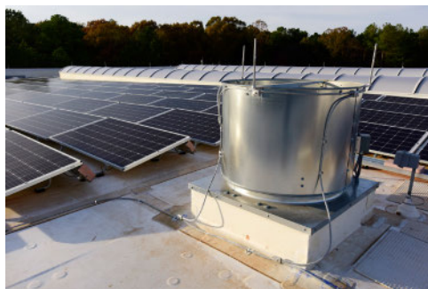
Solar panels generate electricity, rows of translucent panels admit light to the warehouse and exhaust fans ventilate the warehouse space.
